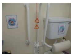
Poor contrast between walls and fittings
